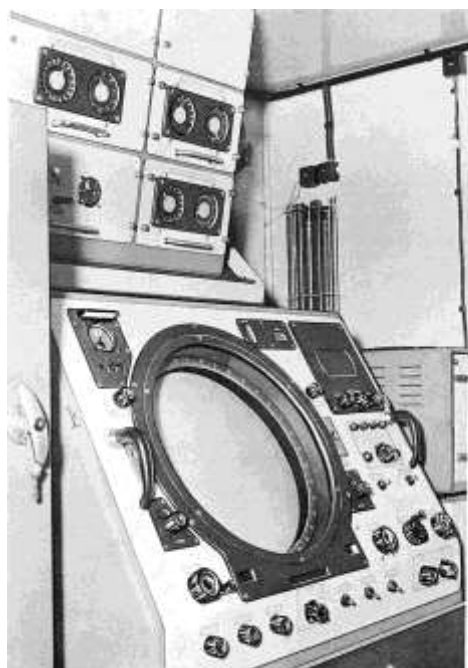
Interior view of a trailer installation, showing the Display Console and Data Presentation Unit.
